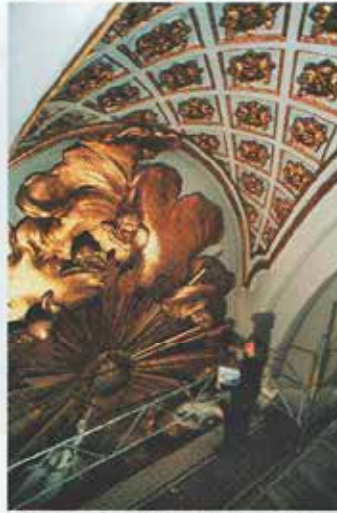
Fig. 6: Condition survey by mapping of the stucco altar in Maria Magdalena church. Photo: H.
