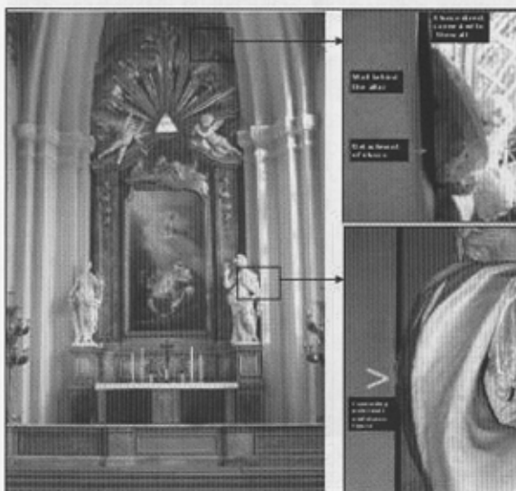
Fig. 1: Examination of the wall-integrated altar in Maria Magdalena church. Zones where the altarpieces have a direct connection to the wall. Photo: A. Henningsson
